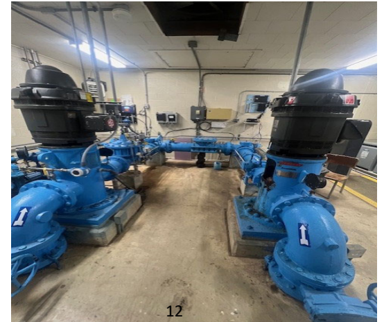
Pump Station interior
