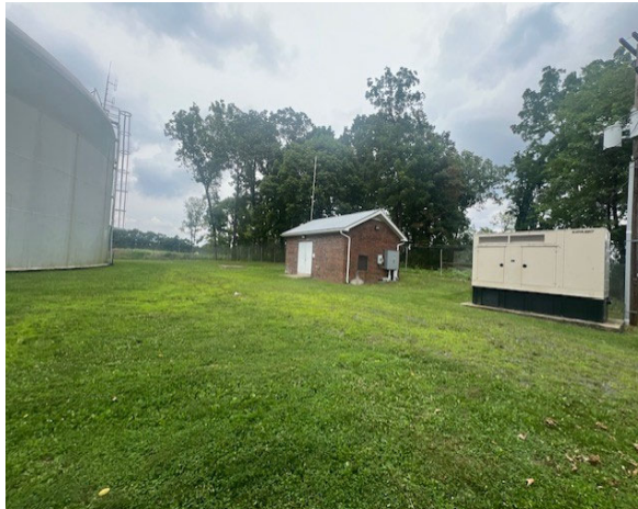
Pump Station with Res. 1 and generator
