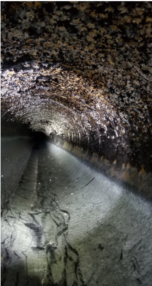
Figure 26 - ARV 8 toward ARV 7 - Blisters in Coating
