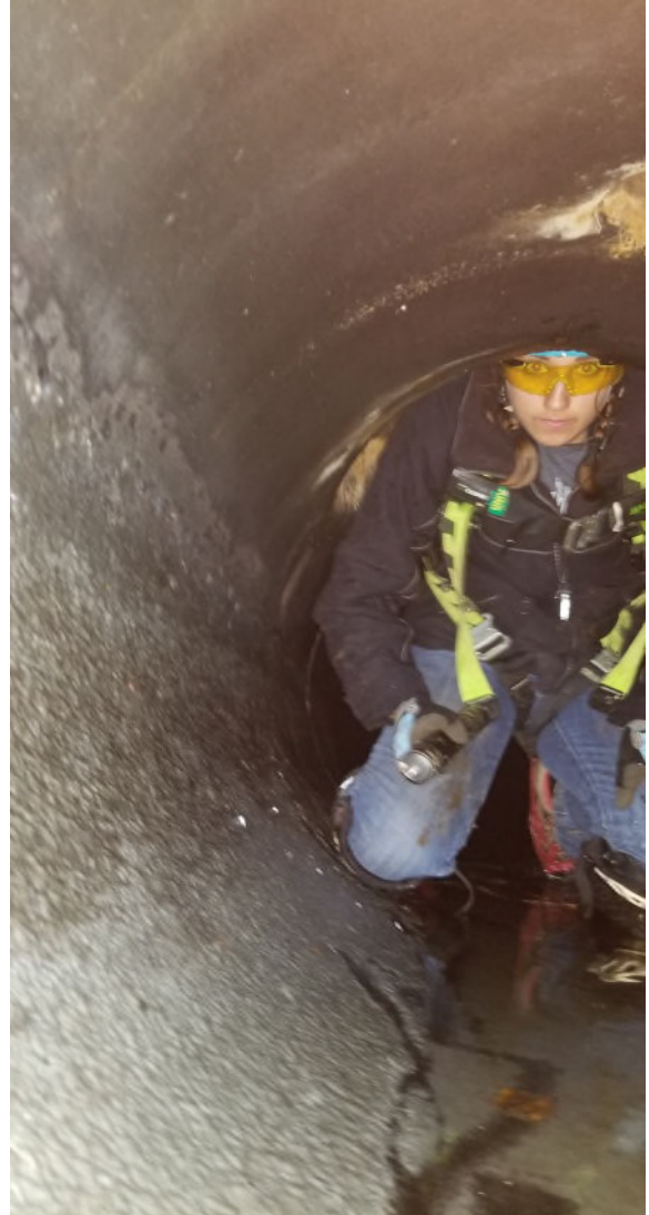
Figure 29 - ARV 9 - ARV 8 Pipe Condition at ARV 9
