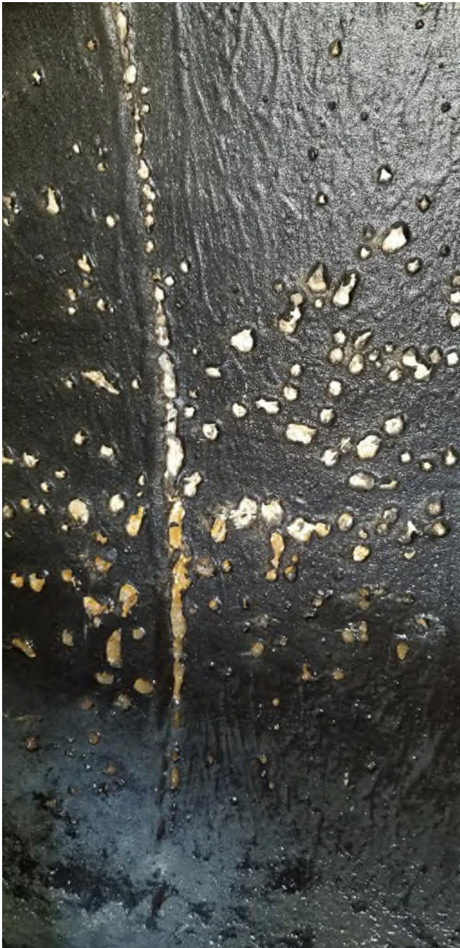
Figure 22 - ARV 6 toward ARV 5 - Coating Blisters and Disbondment
