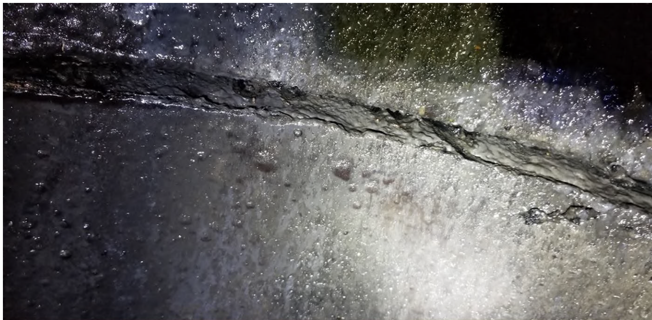
Figure 7 - ARV 5 toward ARV 4 - Unmudded joint
