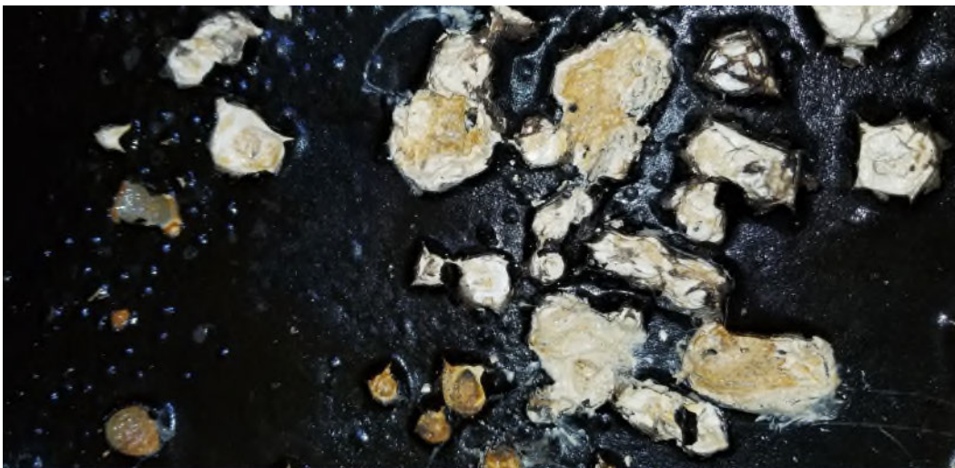
Figure 24 - ARV 6 toward ARV 7 - Blisters in Coating
