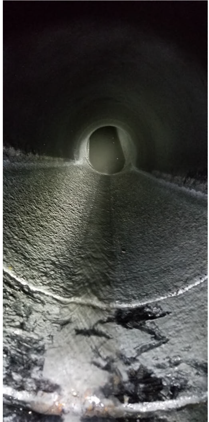
Figure 32 - ARV 9 - Access Chamber 2
