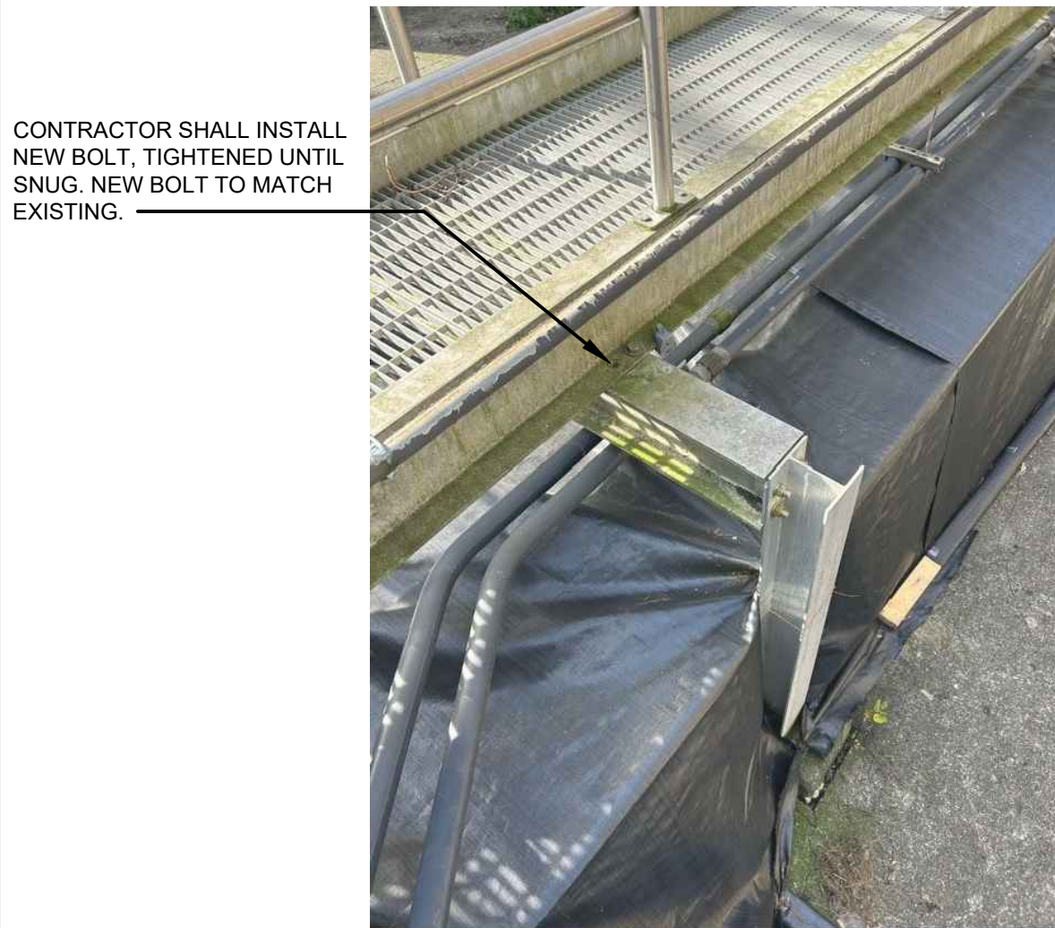
1 PHOTO OF MISSING BOLT SCALE: NONE
