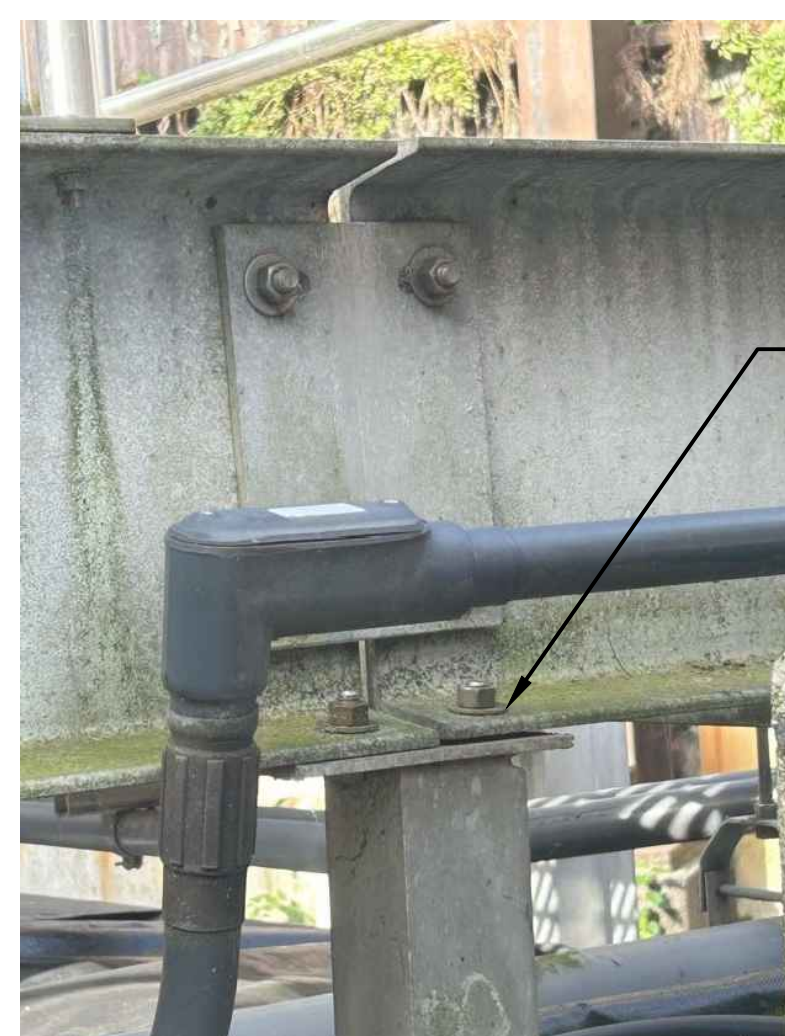
2 PHOTO OF LOOSE BOLT SCALE: NONE
