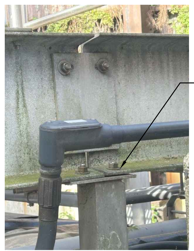
2 PHOTO OF LOOSE BOLT SCALE: NONE
