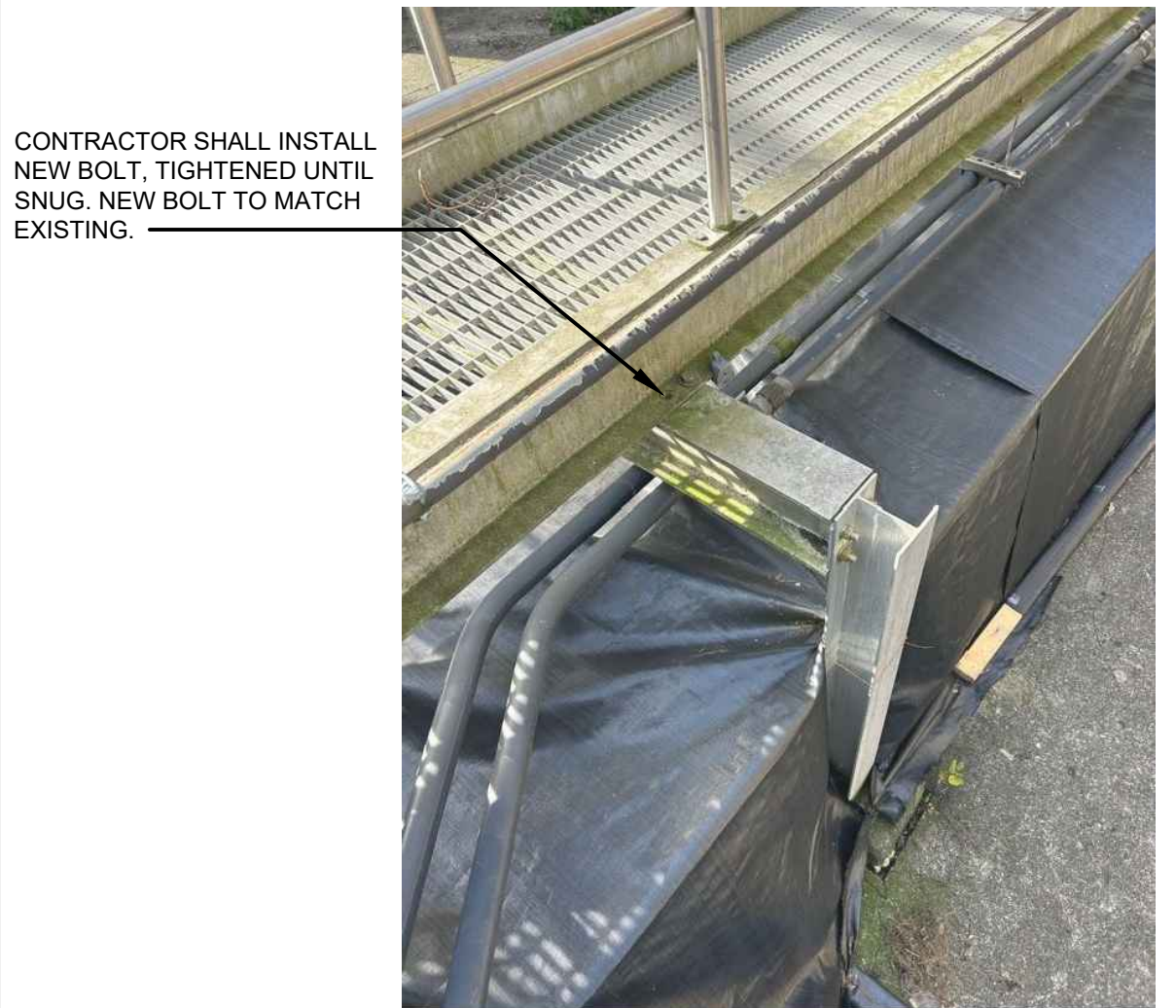
1 PHOTO OF MISSING BOLT SCALE: NONE
